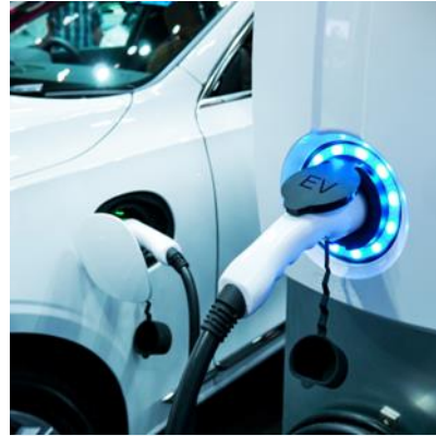
EV charging stations
